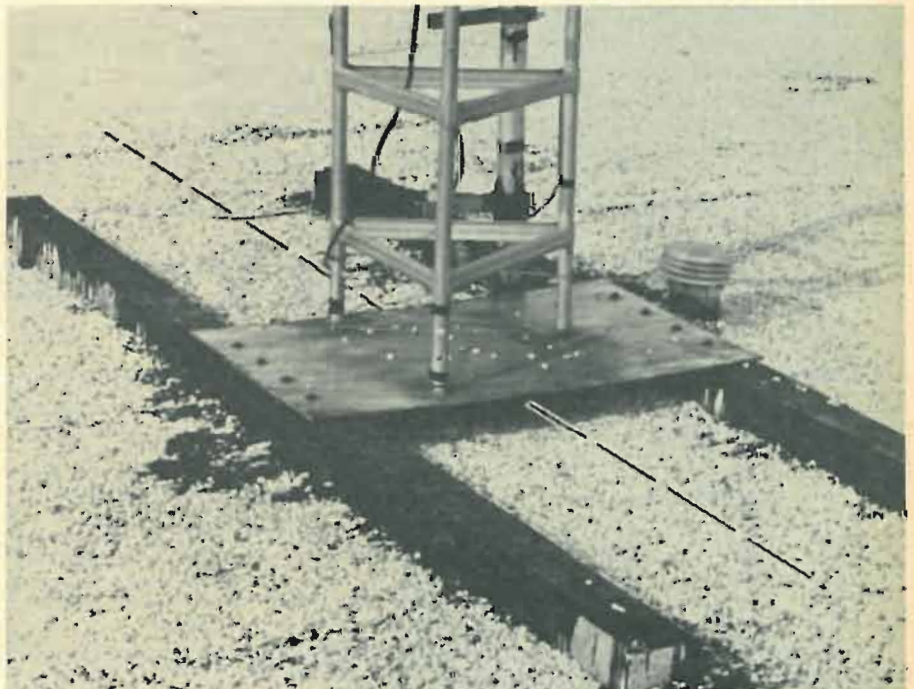
The tower base lies astride a load-bearing wall (indicated by the broken, dashed line) to distribute the tower weight evenly over a major structural member of the roof itself.
